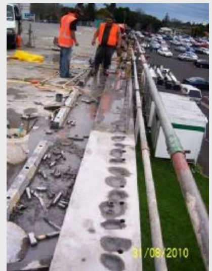
Work continues on adding two more levels to the multi-storey car park
