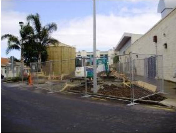
A new annexe is being built outside the Kidz First main entrance
