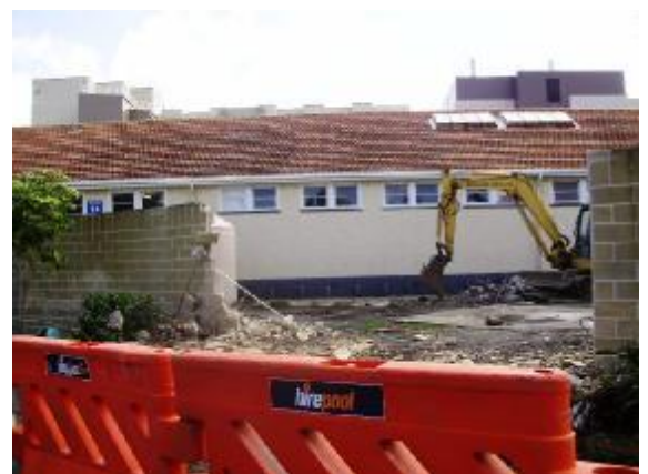
The hole in the wall will provide vehicle access to the Kitchen and Inwards Goods
