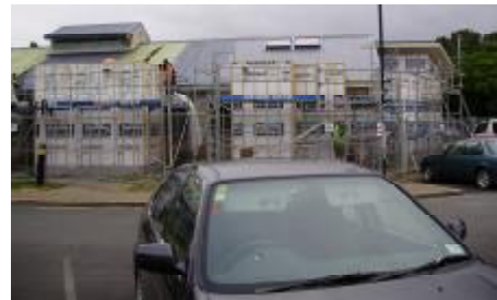
In the next few weeks you'll see the walls going up for the new ensuites
