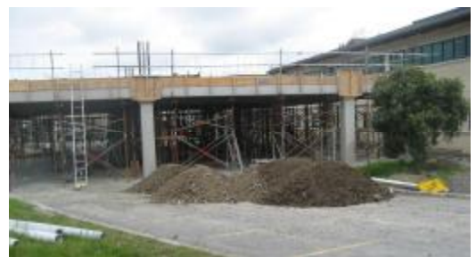
Construction of the new Ophthalmology Outpatient Department on the Ground Floor, Building A.
