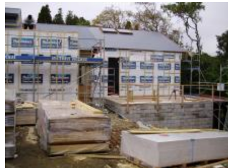
A secure courtyard will be attached to the ICA. Note the skylights in the ICA Roof.
