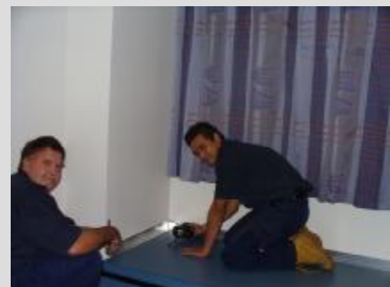
Carpenters Mike (left) and Sao carry out repairs to Kidz First Surgical.
